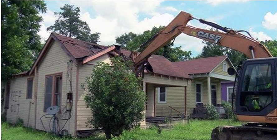
The Blight Strike Team demolishing an abandoned property in East Baton Rouge Parish
